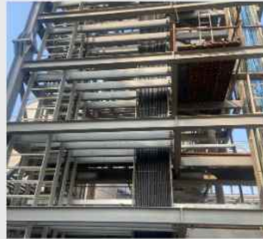
HPCL-MITTAL ENERGY LIMITED (HMEL): BHATINDA
