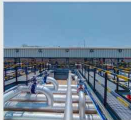
NATIONAL THERMAL POWER CORPORATION (NTPC): RAMAM
